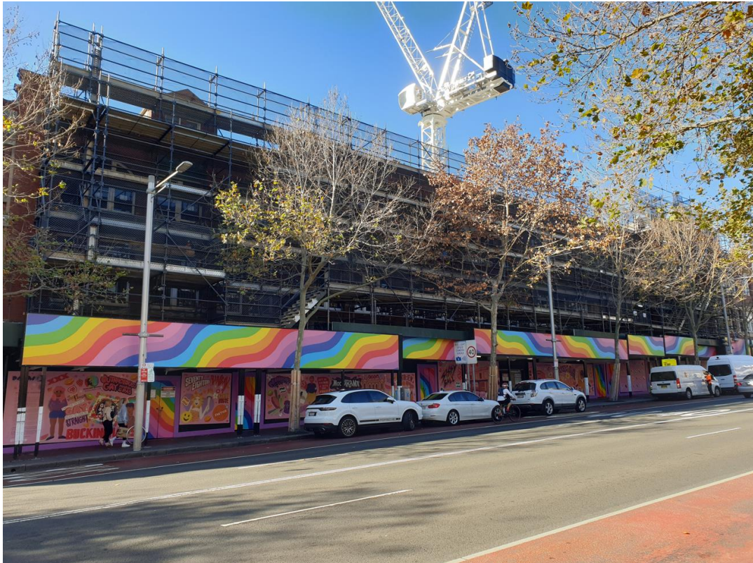
Figure 13: The buildings at 58-78 Oxford Street, Darlinghurst, viewed from the south-western side of Oxford Street, looking east
